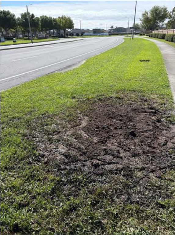
Mainline leak along Ayersworth
